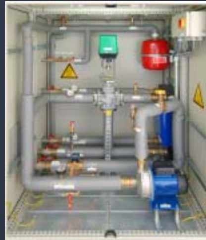
Cooling water heat exchanger
